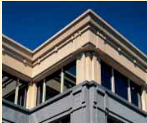
Leaf North America's Corporate Headquarters in Lake Forest, Ill., features a distinctive limestone-finished stepped cornice. The design element, articulated with triglyphs over each column and dentil moldings between, provided an economical way to give prominence to this suburban office building. Photos: George Lambros Photography
